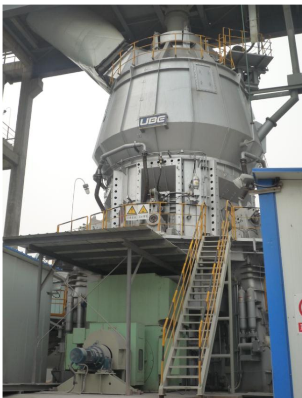
Fig. 4 Slag Grinding Plant and 6 Roller Mill
